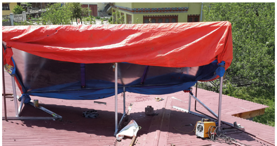
Solar collectors being installed on the roof of a hotel in Bhutan
